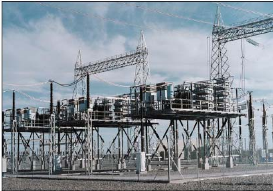
Series capacitors, 215 Mvar, 500 kV, Argentina.
