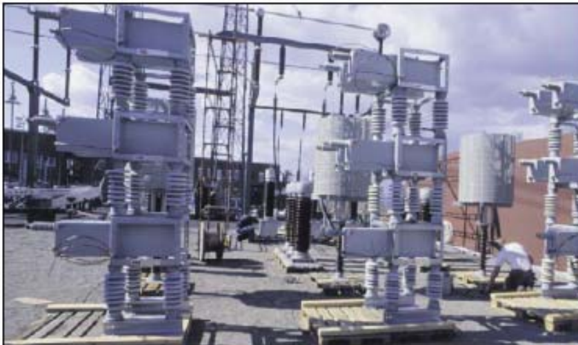
HVDC Light, Gotland, Sweden.
